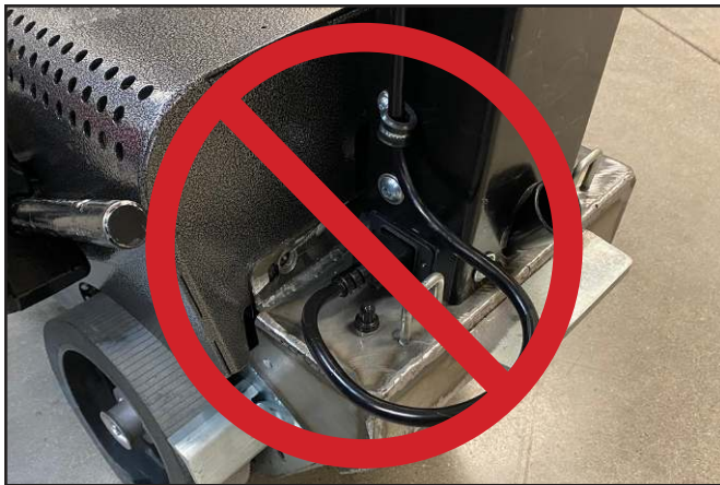
Power cord should NOT have excess slack.
